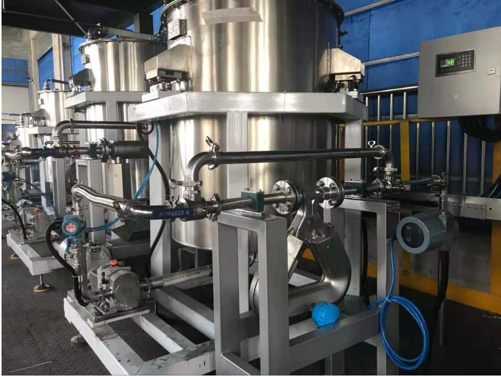
Example Two: The Alpha mass flowmeters are installed inside a chemical plant for the raw chemical material process measurement.
