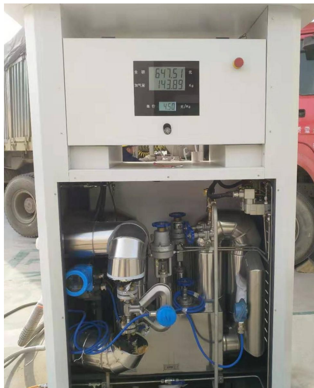
Example Three: An Alpha mass flowmeter is installed in a gas station for the fuel measurement.
