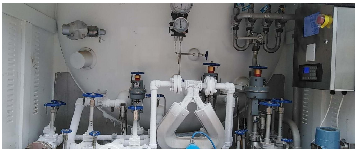
Example One: An Alpha mass flowmeter is installed in a truck-loading cryogenic system for batch operation.
